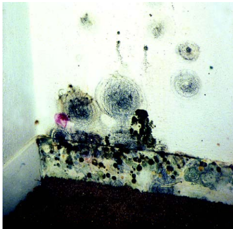
Photo 3A: Mold growing in closet as a result of condensation from room air
